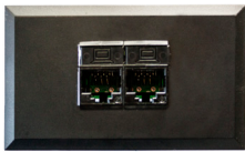
2 RJ45s (data/network connectors) in one opening
